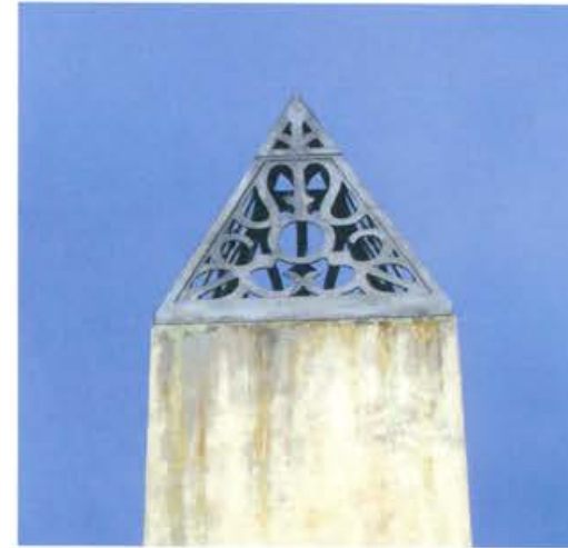
Ventilation system in Hyde Park Obelisk
