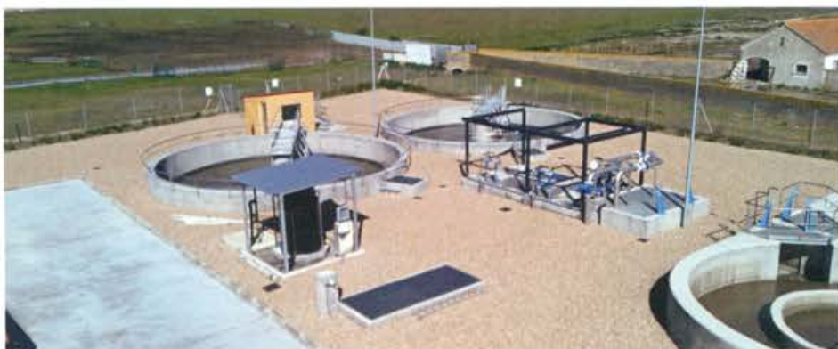
Water treatment plant, Olmedo, Valladolid. 2015
