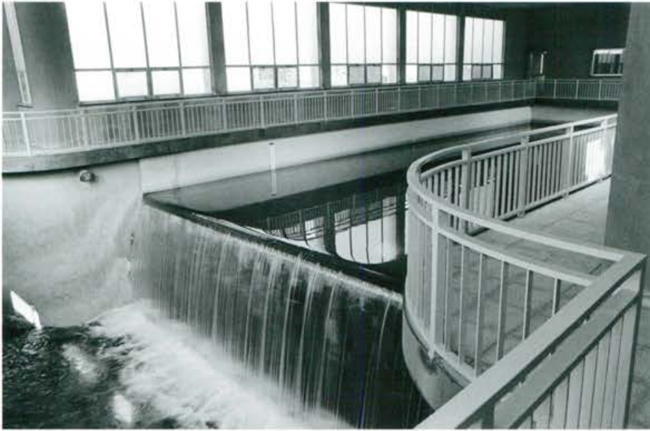
Entry of water to the lower tank at Plaza de Castilla
