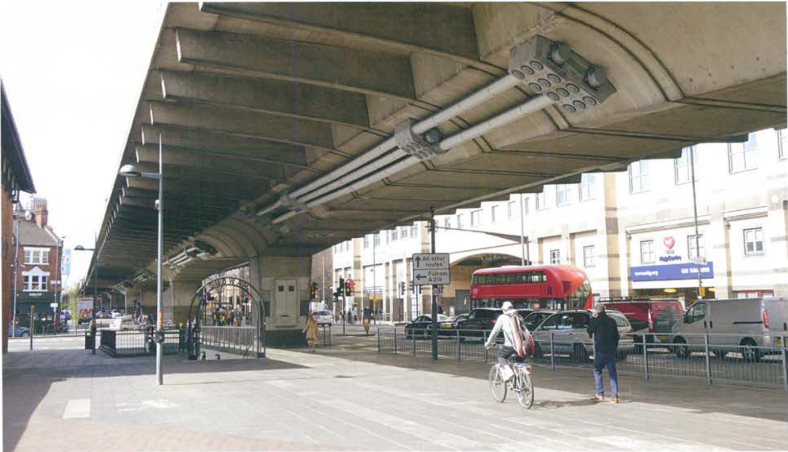
Hammersmith Flyover for the accesses to Heathrow, designed by G. Maunsell & Partners, and built in 1961 by prefabricated elements sewn with post-tensioned cables and later reinforced in 2011 with additional external cables to supplement the interiors, attacked by water filtrations.
