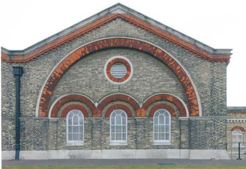
Crossness Pumping Station
